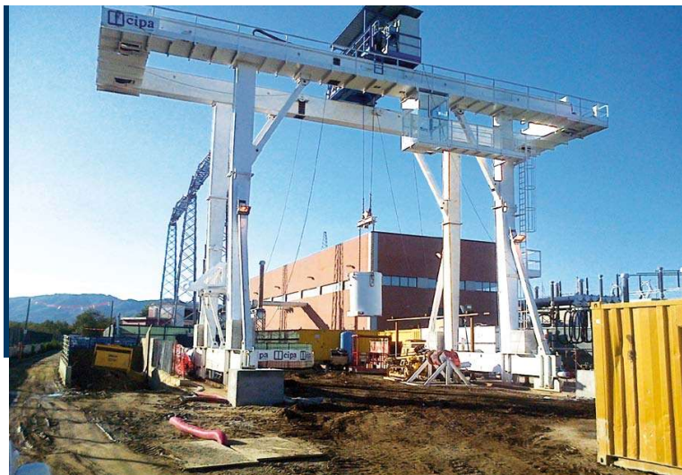
Installation du chantier Melia - Pont roulant Installation of Melia work site - Crane
