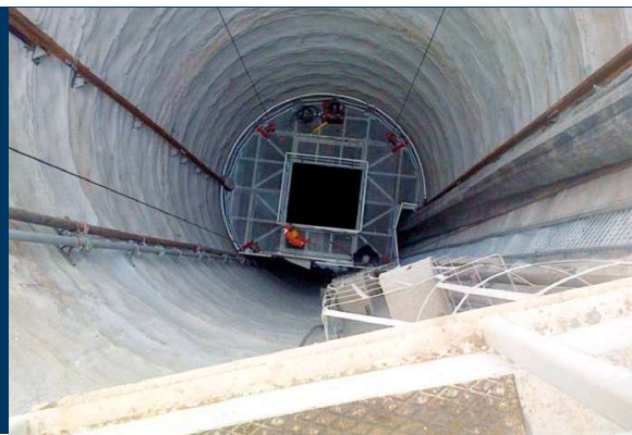
Installation du chantier Melia - Plate-forme de service Installation of Melia work site - Service platform
