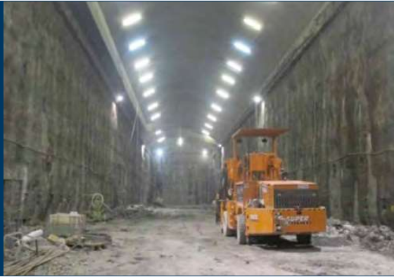
□ Image des cavernes pendant les étapes de banc successives □ Image of the Cavern during the successive bench steps
